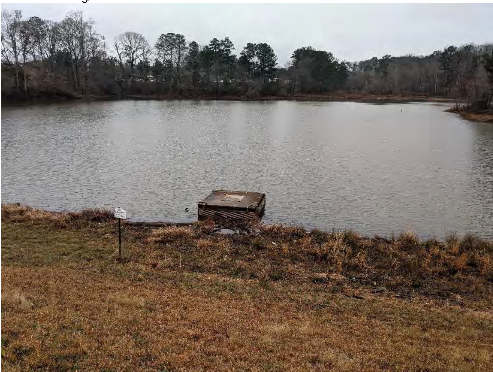
Photo 16: View of outlet control structure located on southern portion of Nelson Pond.
