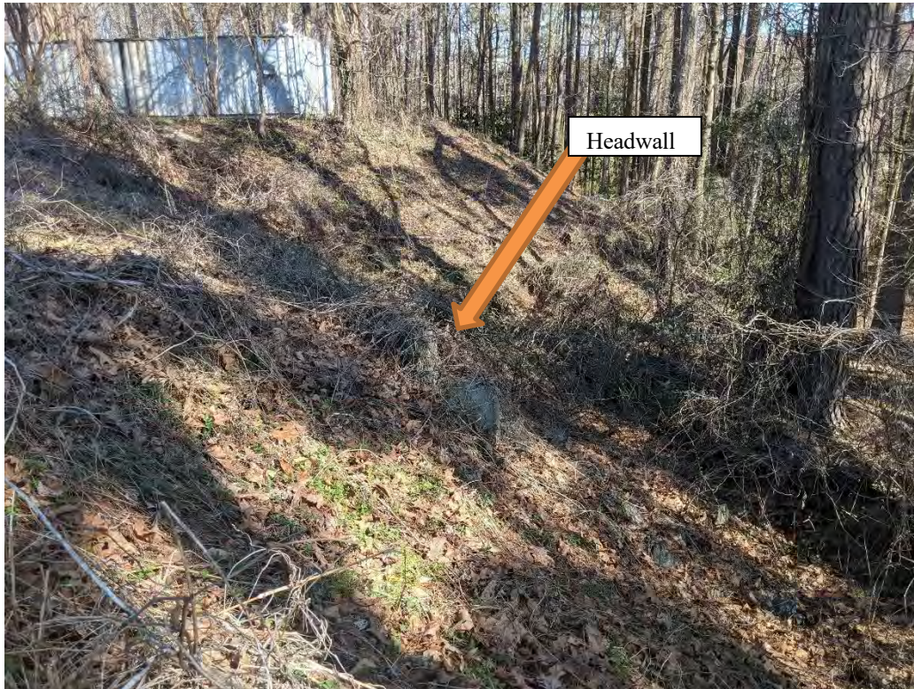
Photo 15: View of SW-M13 (headwall) located south of the Gymnasium and Lot P21.
