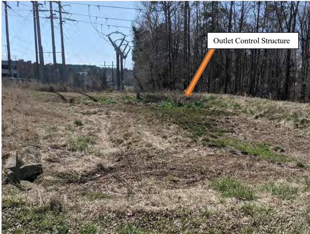
Photo 25: View of detention pond and outlet control structure (OCS8053) discharging to SW-M21 located near Facilities building.
