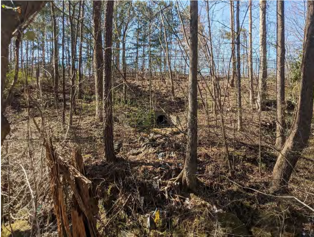
Photo 23: View of SW-M20 (headwall) east of Technology way and south of Lot P11.
