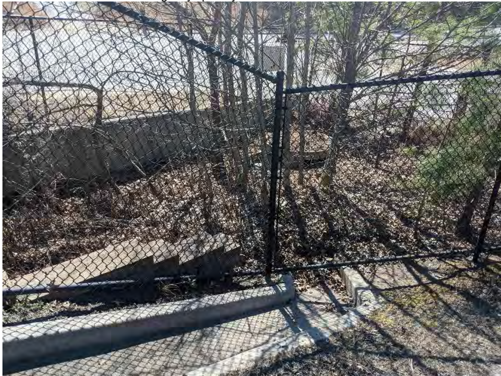
Photo 20: View of wier inlet located in the south side of the Perch entrance drive. Discharges to SW-K13.
