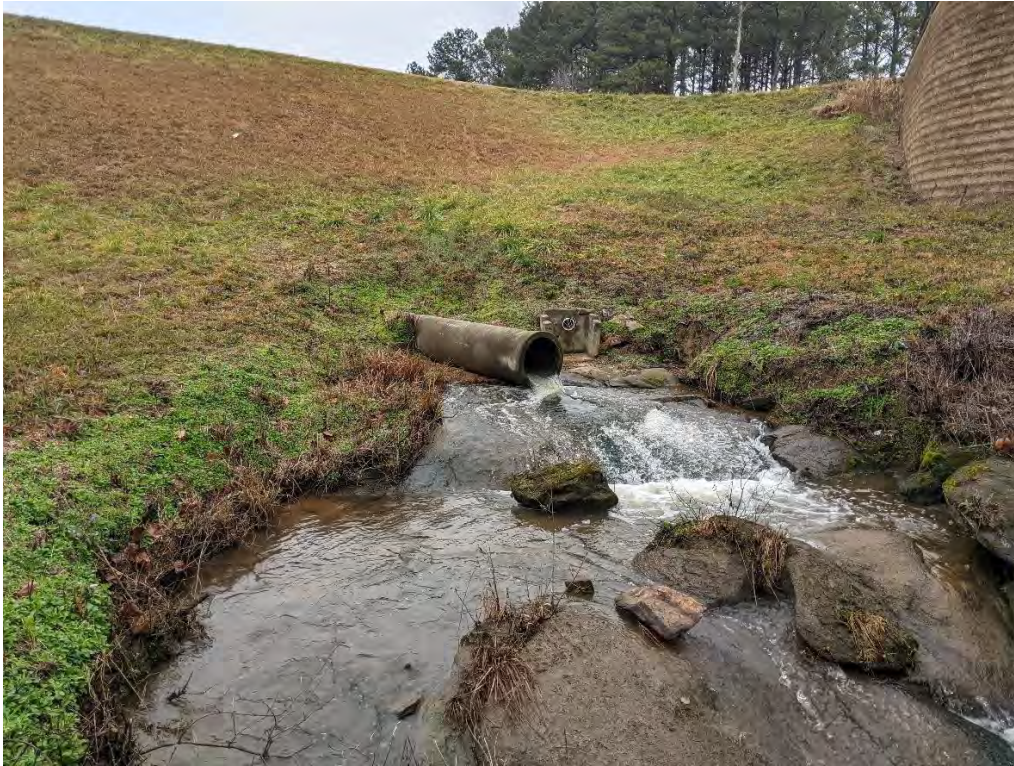
Photo 17: View discharge from outlet control structure within Nelson Pond, located on south side of the Category1 dam.
