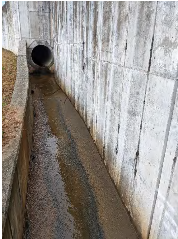
Photo 19: View of concrete pipe discharging into concrete channel located on southern portion of Nelson Pond emergency spillway.
